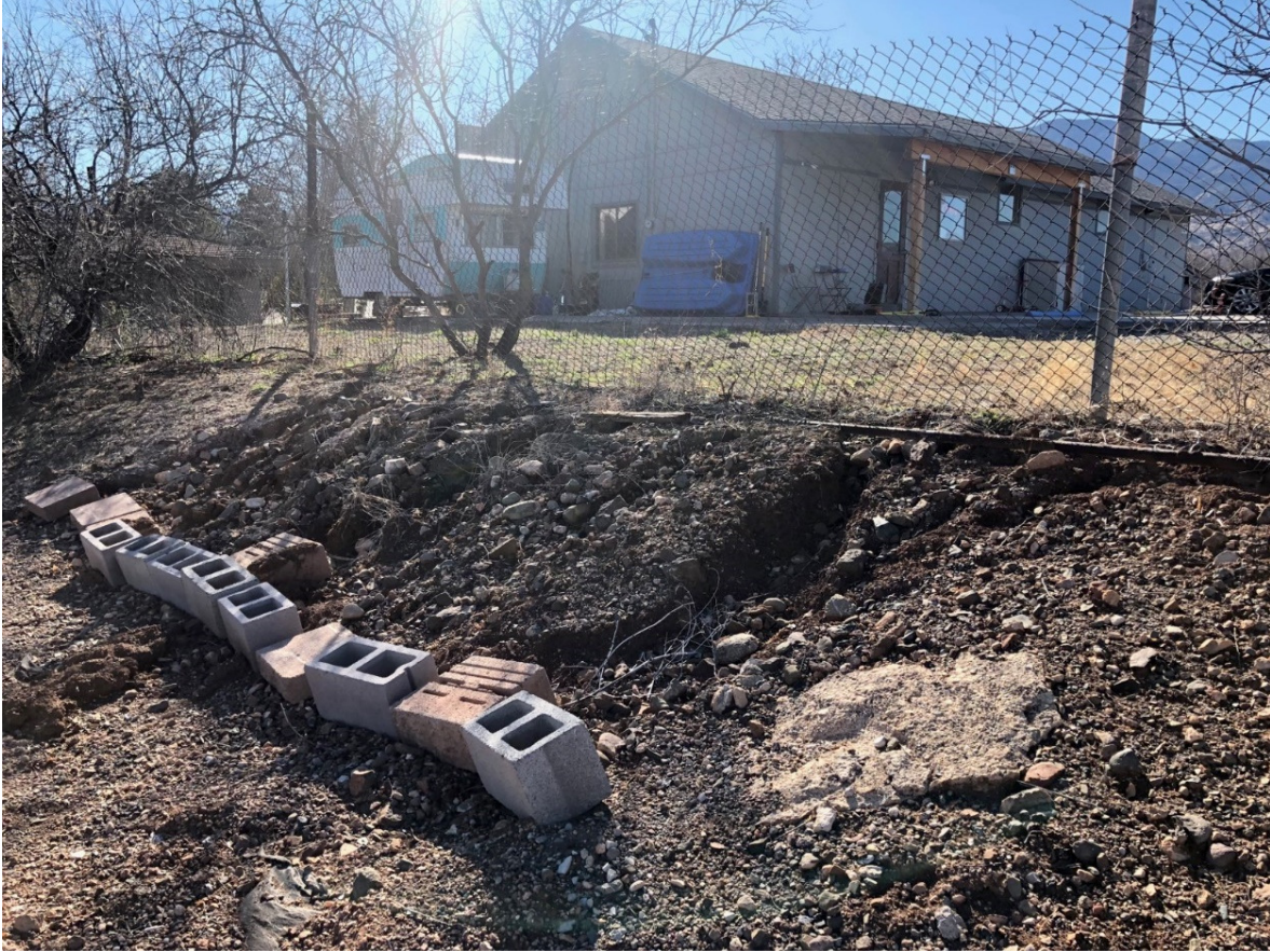
Figure 3. Erosion Occurring on Site
